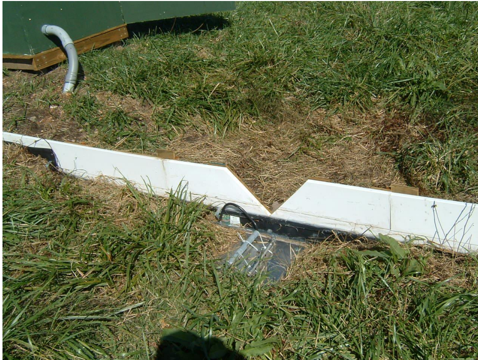
Photo 7. V-Notch Weir, Pressure Transducer, and Strainer Location
