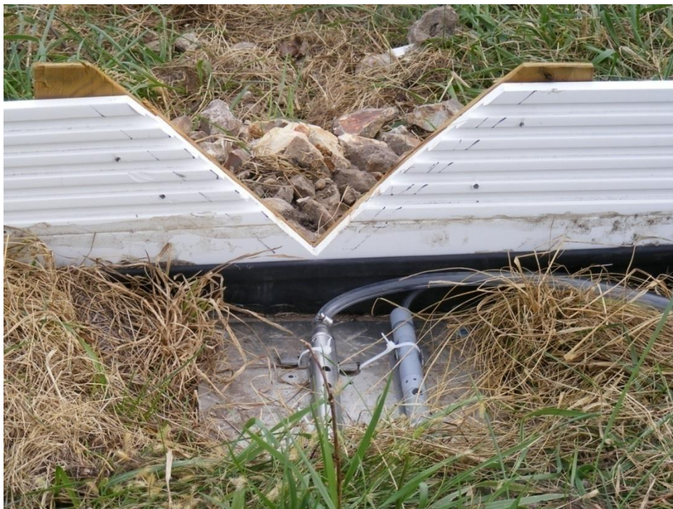
Photo 8. Pressure Transducer and Strainer Location
