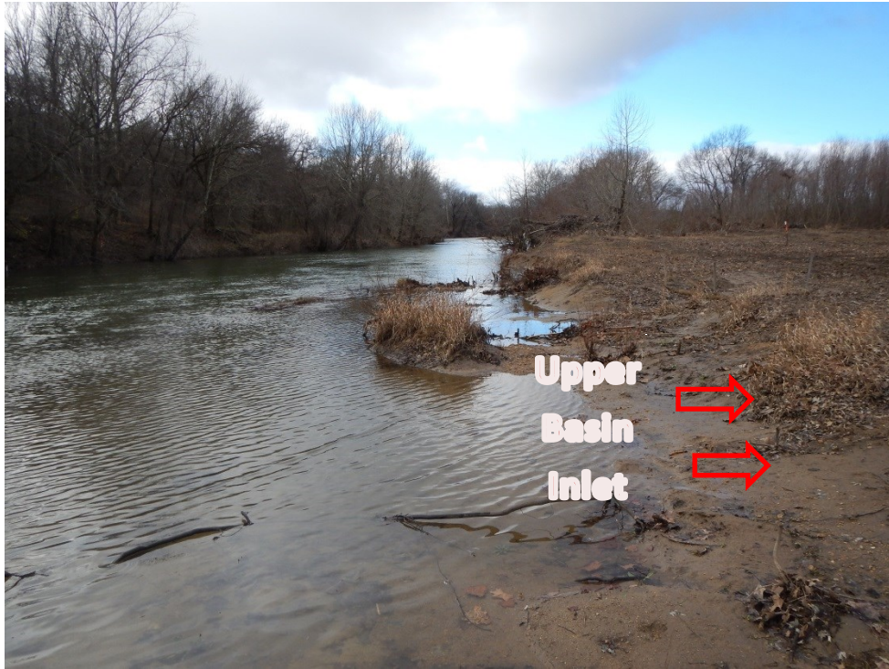
Photo 11. Lowered bank at the upper basin inlet experiencing erosion after several large flood events, upper basin inlet to the right (12/14/15).
