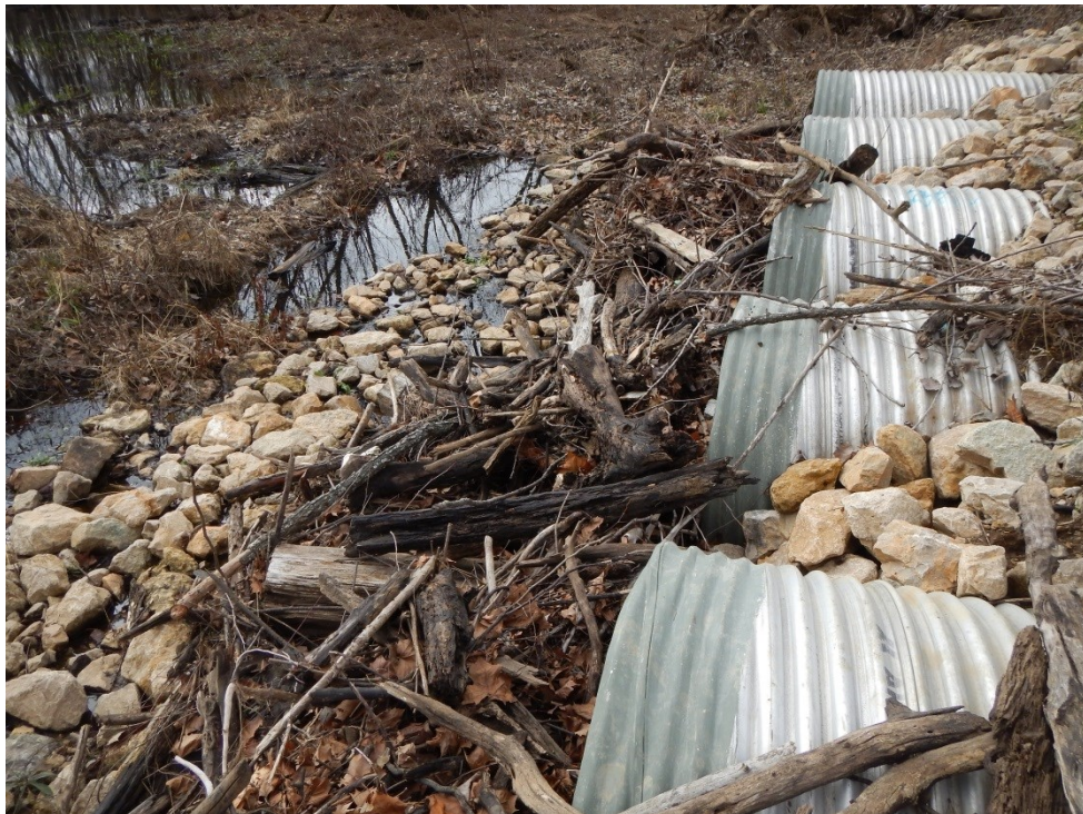
Photo 12. Debris jam blocking lower basin secondary outlet (12/14/15).
