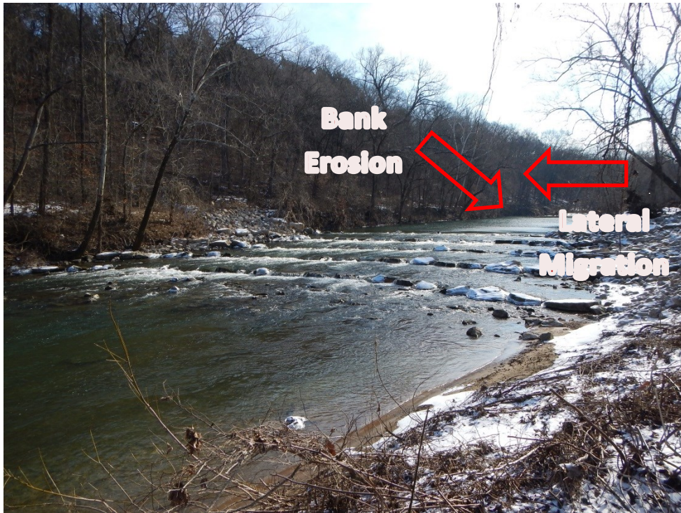
Photo 9. Riffle structure creates high water situation that could weaken bank over time and increase erosion (1/21/16).
