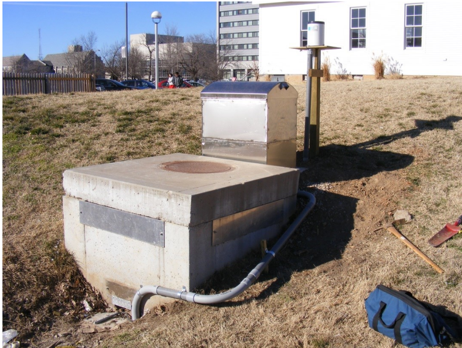
Photo 6. Complete installation of monitoring station with pressure transducer, pump tube, rain gage and stainless steel box
