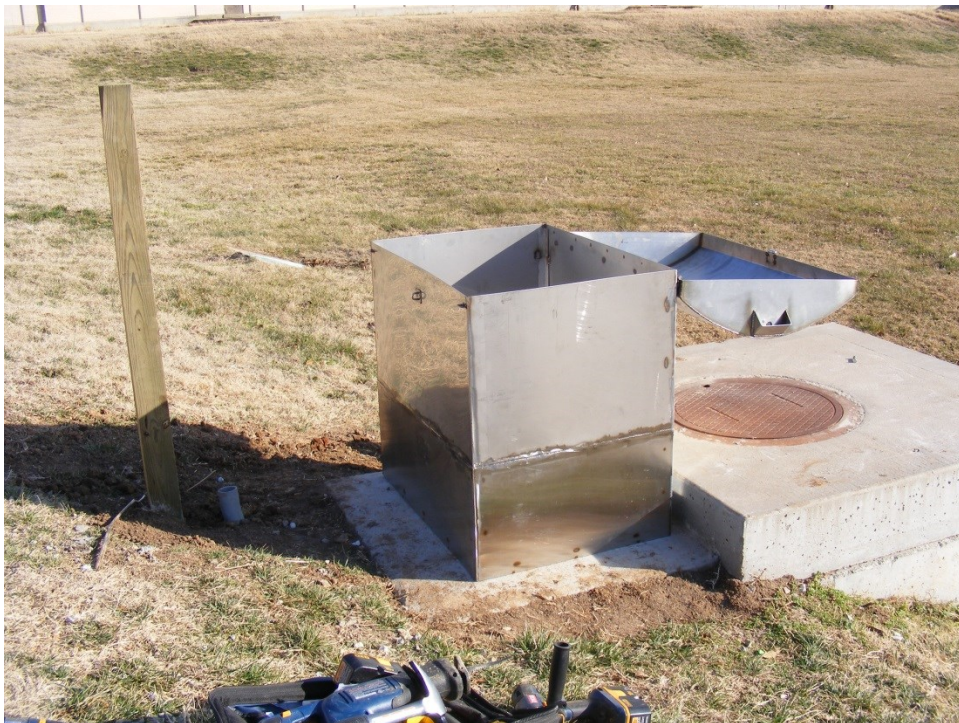
Photo 4. Stainless steel box secured to concrete pad with rain gage post installed
