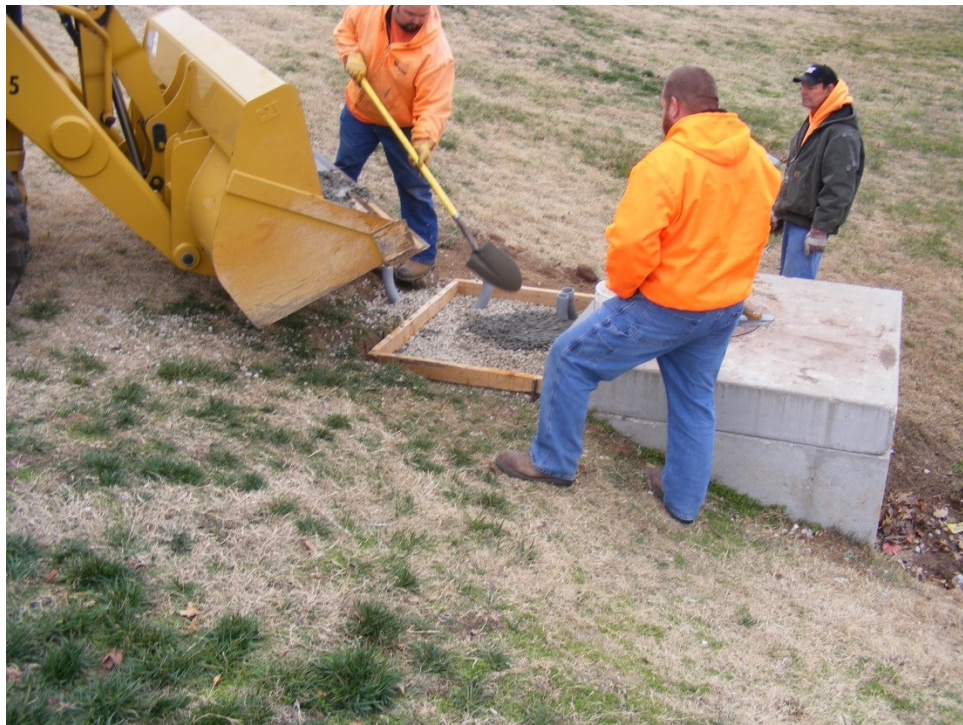
Photo 2. Pipe rough in, concrete forms and pad pouring by City of Springfield crews
