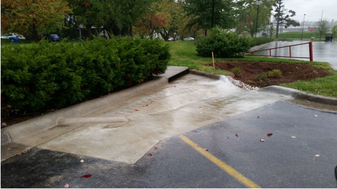
Photo 9. Rain garden installed in the parking lot draining to the Drury basin
