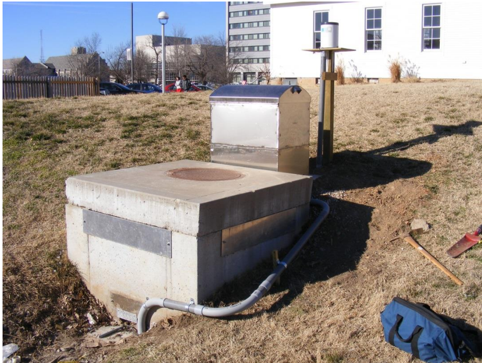
Photo 6. Complete installation of monitoring station with pressure transducer, pump tube, rain gage and stainless steel box
