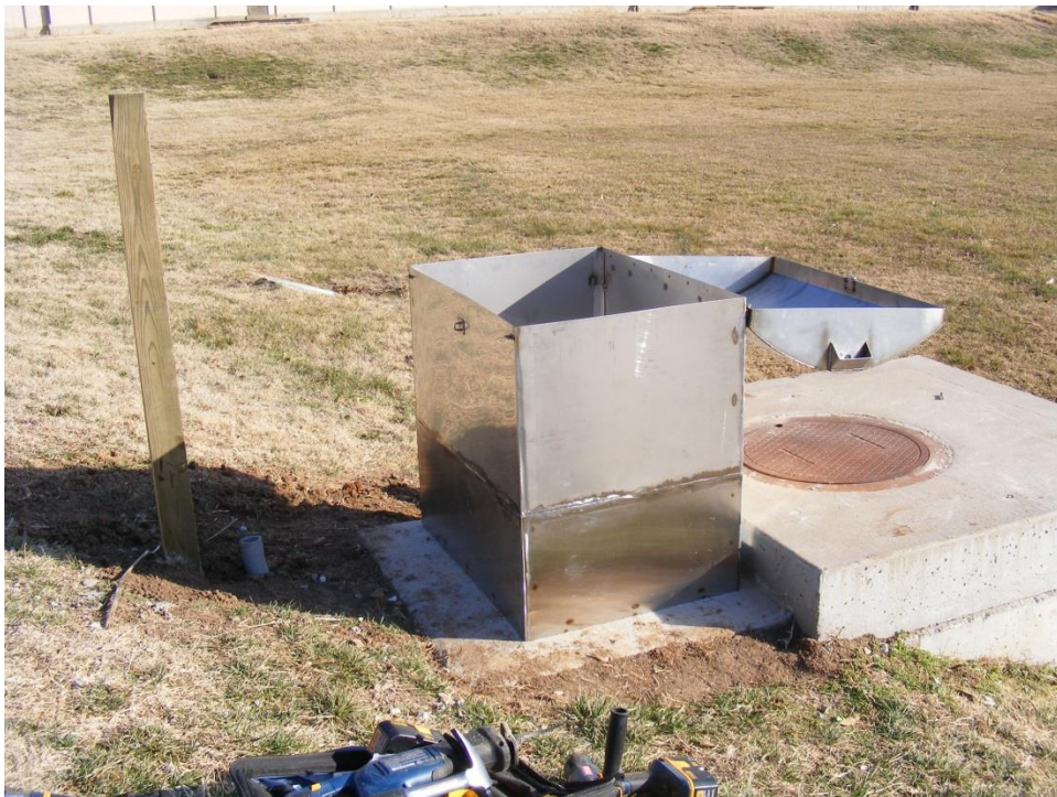
Photo 4. Stainless steel box secured to concrete pad with rain gage post installed
