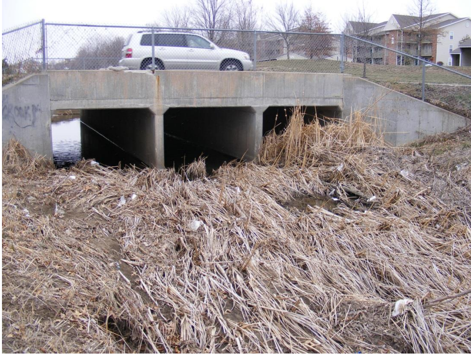
Photo 9. Example of problem type 9. Sedimentation inside culvert decreasing flow capacity.
