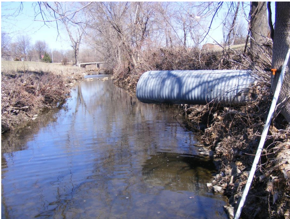
Photo 8. Example of problem type 8. Hanging culvert or inlet due to incision.
