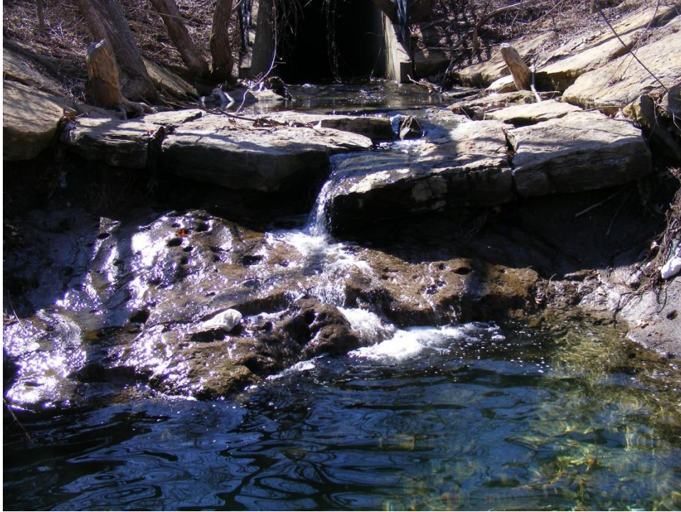
Photo 5. Example of problem type 5. Bed erosion/undermining at bridge
