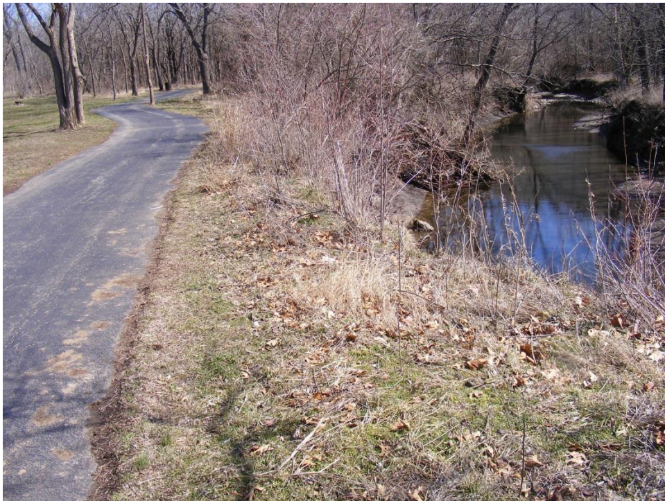
Photo 2. Example of problem type 2. Bank erosion and failure risk-greenway trail
