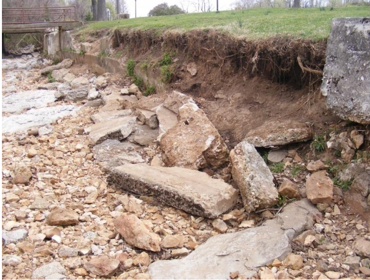
Photo 26. Failing concrete wall on right bank looking downstream near station 1,200 feet SR-3 (4/6/09)
