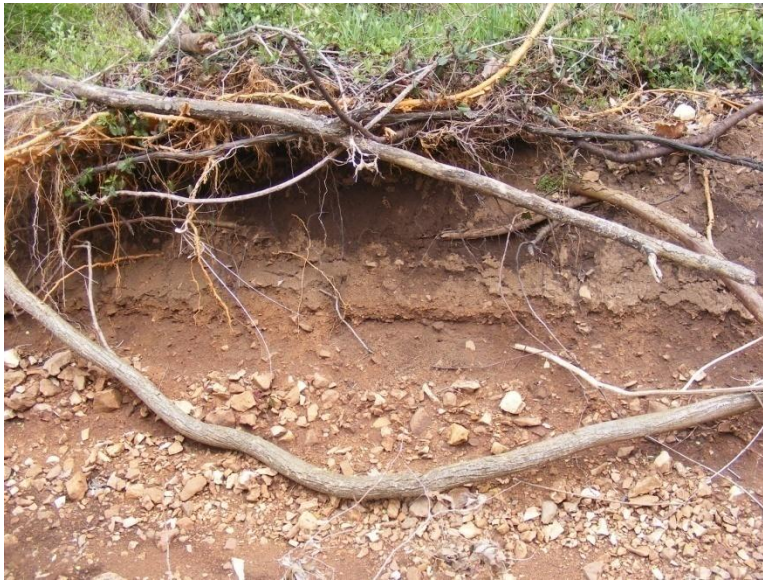
Photo 20. Bank erosion downstream of Lacuna bridge in reference reach B (4/6/09)
