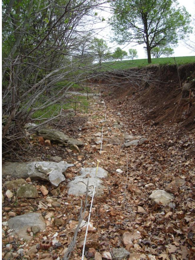
Picture 3 – Bedrock exposure and bank artifacts on the right side at 600ft (sub-reach #1)
