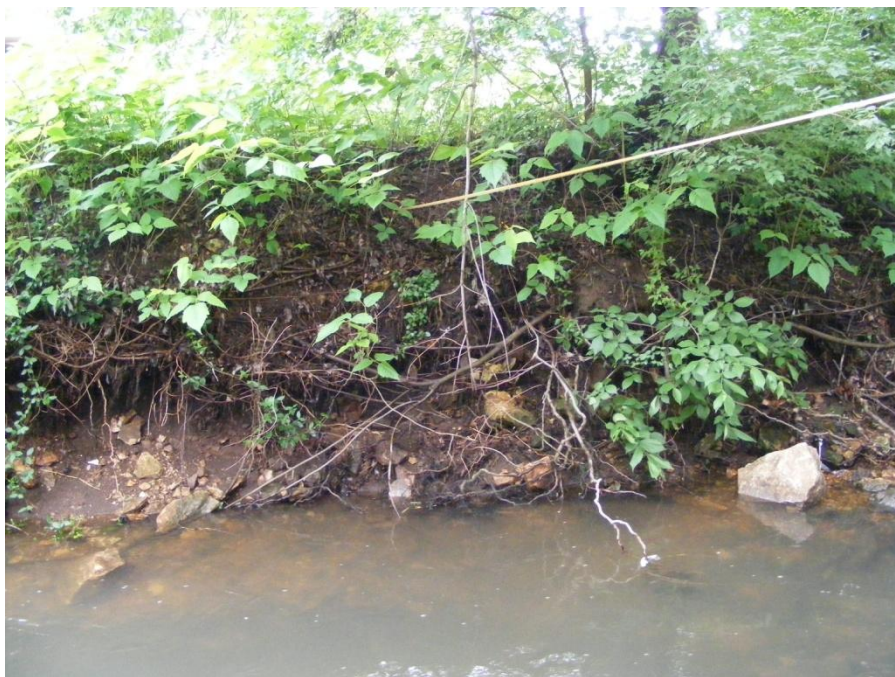
Photo 58. SR-15 section #9 (station 3,875 ft) left bank.
