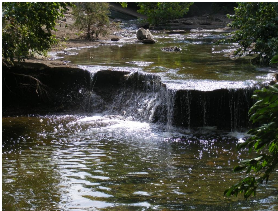
Photo 60. SR-15 scour hole below concrete apron appears to be supported by compacted cherty-clay fill material that is being undercut (station 4,025 ft).
