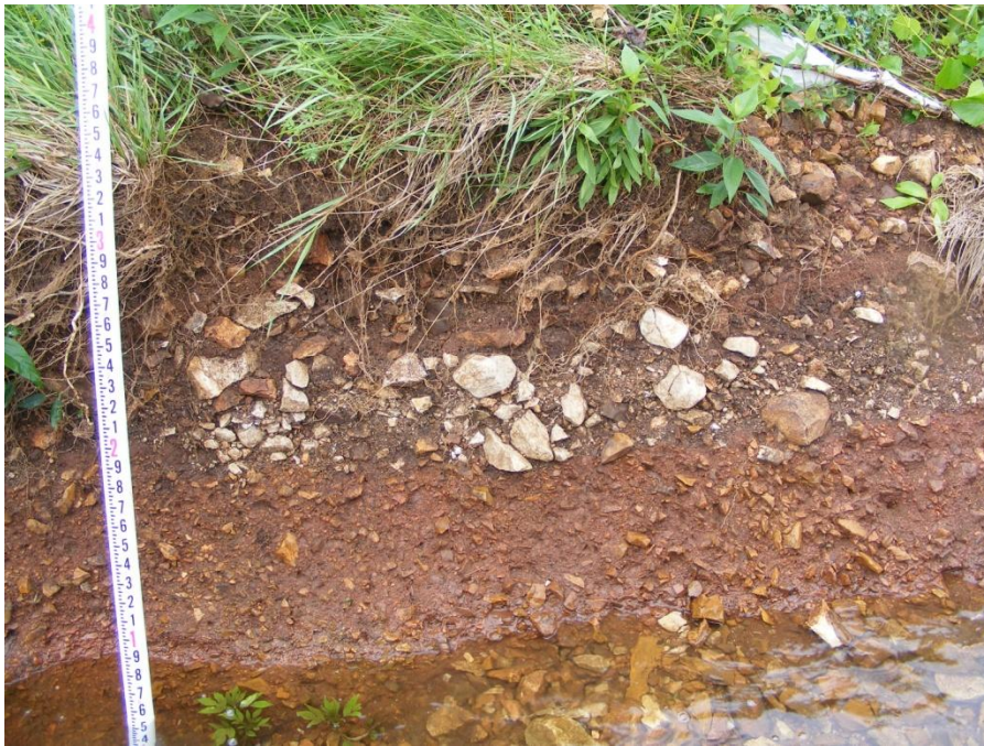
Photo 34. SR-9a bank erosion at station 1,500 ft.
