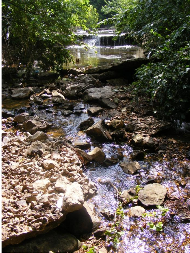
Photo 59. SR-15 looking upstream toward the Bradford Lake spillway with busted pieces of concrete in the channel downstream of the scour hole below the apron (station 3,940 ft).
