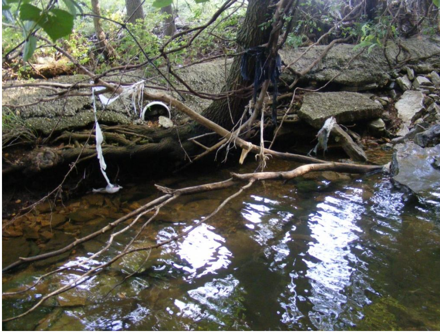
Photo 19. SR-5 undercut concrete sewer casing starting to fail (station 750 ft)
