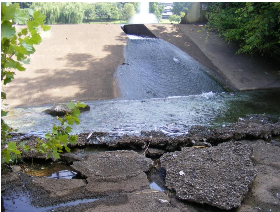
Photo 62. SR-15 downstream of Bradford Lake outlet structure concrete slabs are being pulled off the floor of the spillway.
