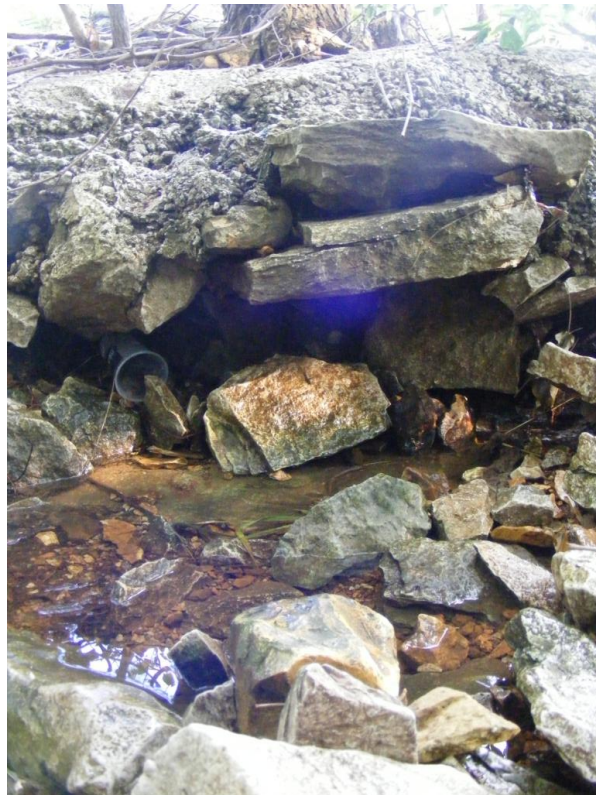
Photo 20. Unconsolidated material supporting sewer casing is washing away (station 750 ft)
