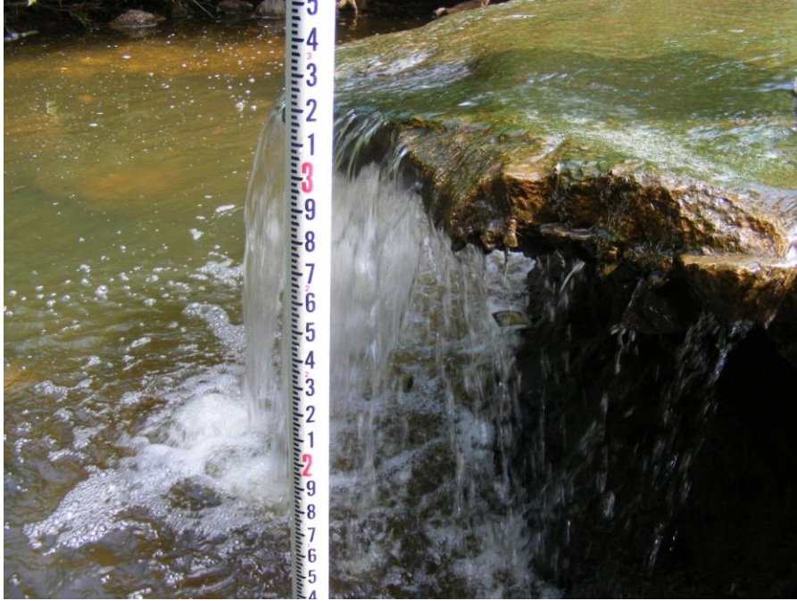
Photo 61. SR-15 concrete apron of spillway is undercut around 3 ft (station 4,025 ft).
