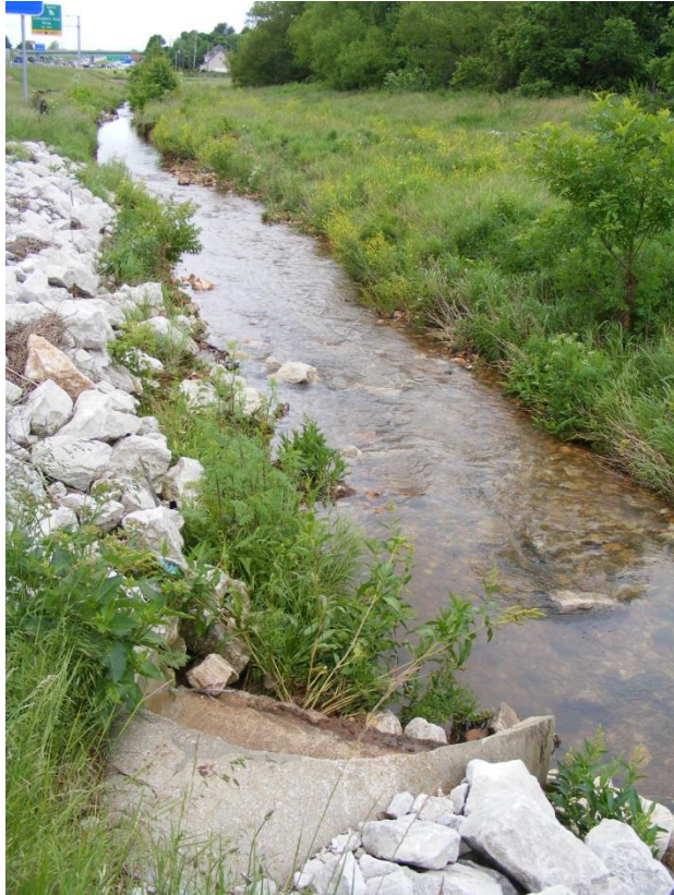
Photo 39. SR-10a located below storm pipe at station 1,840 ft.
