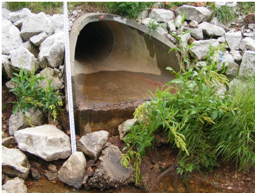
Photo 40. SR-10a local scour around storm pipe outfall at station 1,840 ft.
