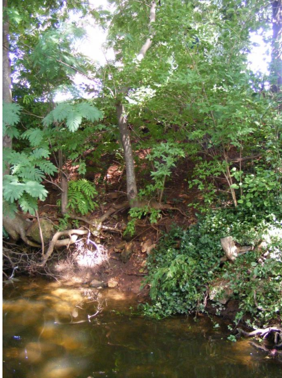
Photo 53. SR-15 right bank erosion and slump along Bradford Parkway (station 3,825 ft)
