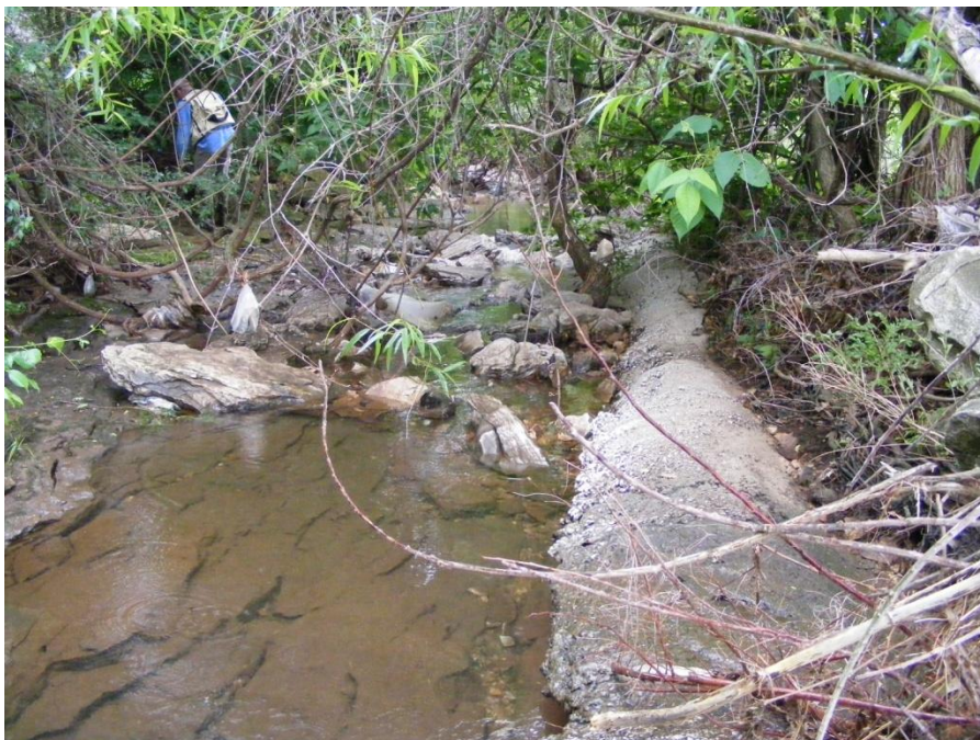
Photo 22. SR-5 sewer line casing exposed along right bank through bedrock knick point assemblage. Stream is cutting north (right bank) that will continue to expose more of the sewer line (station 830 ft).
