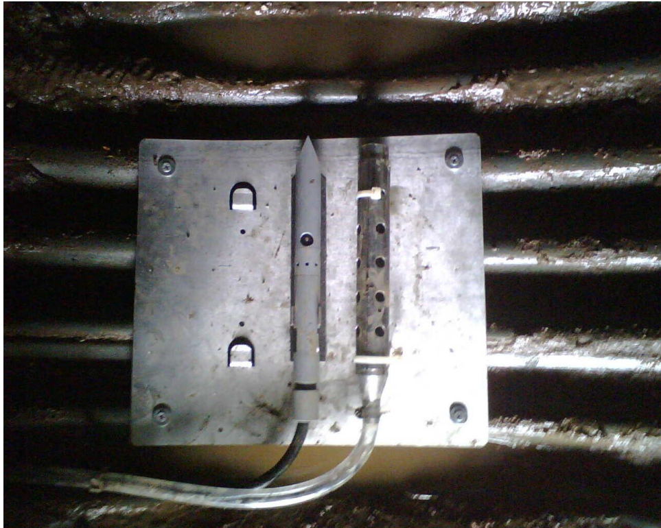
Photo 6. Mounted Pressure Transducer and Strainer in Pipe Invert
