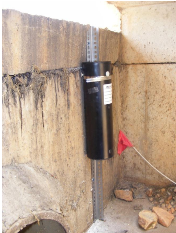
Photo 10. Curb inlet sampler installed at Park Hill
