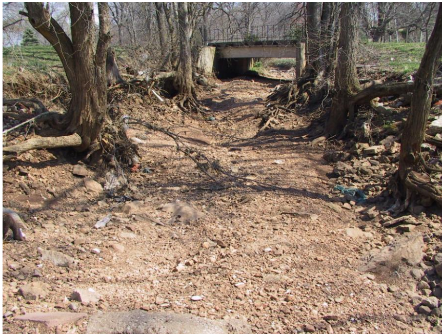
Photo 4. Scour hole at station 2,100 feet
