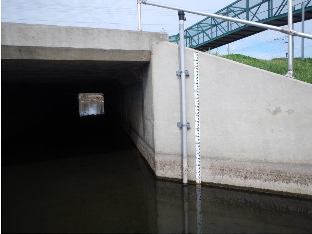
Photo 5. Levellogger and staff gage installed at KAN.
