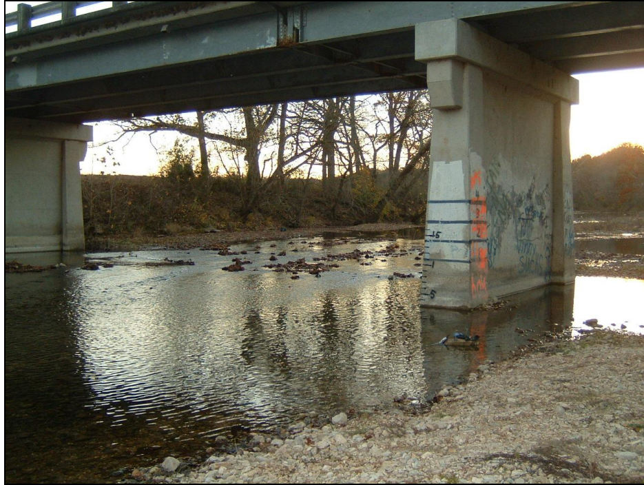
Figure 2.19: Bear Creek (19). Site at Highway 14 Omaha, AR (November 13, 2005)
