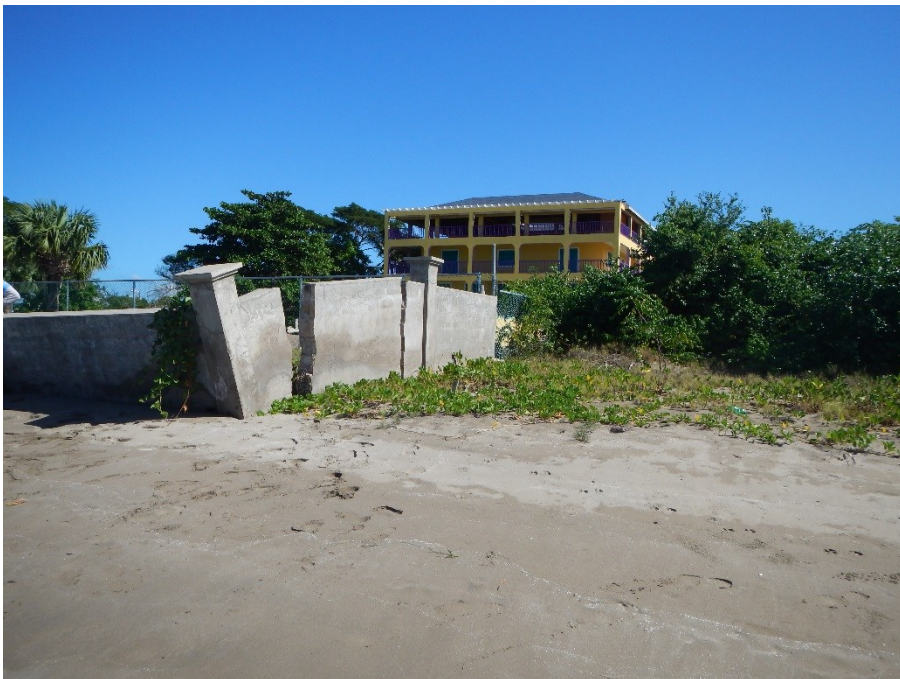
Damaged infrastructure (transect 440).
