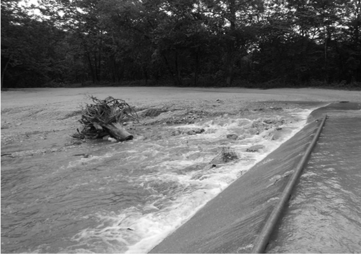
Figure 4. Image of the lateral overflow formed along the edge of the main channel crossing during moderate flows. The discharge at Akers Ferry was approximately 28 \text{ m}^3/\text{s} during this photo. Photo taken 17 August 2017.
