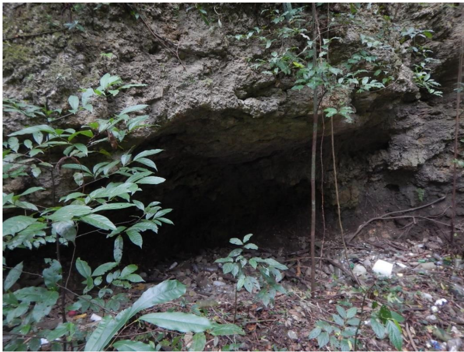
Appendix B-20. Point 17 – A “Scour Cave” on the Wall of the Brighton-Blue Hole Gorge Is an Erosional Feature Which Indicates the Removal of Wall Material Along Fractures
